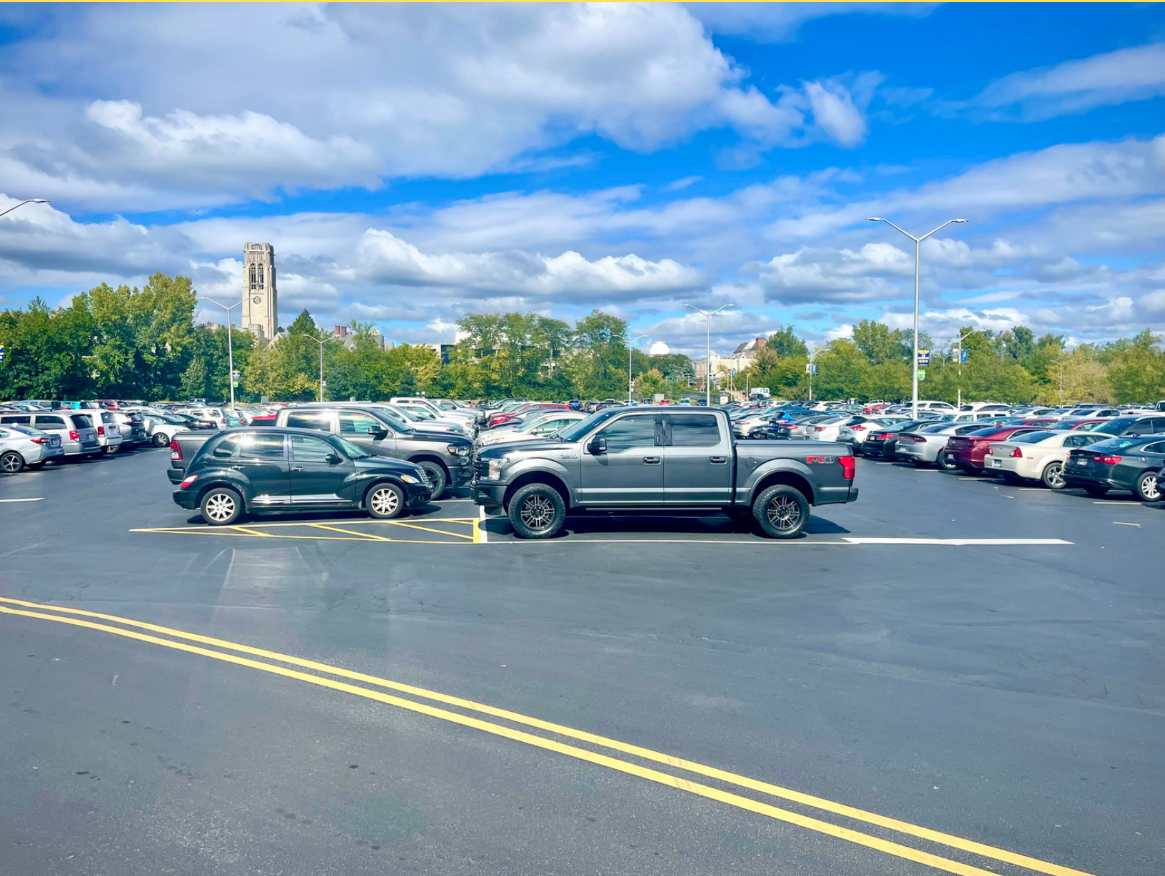
Area 10 - Freshly ressealed and restriped surface lot located along Stadium Drive just North of the Glass Bowl.
